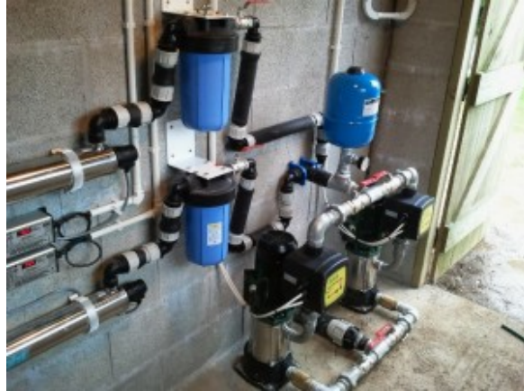
Filtration and Pumping
