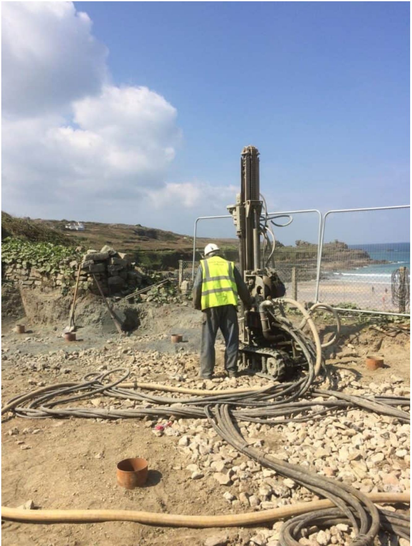
Aquasource SW Ltd has been piling at Porthmear Beach, St Ives for a new build house.
