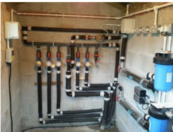
Commercial Water Manifold installation in Cornwall
