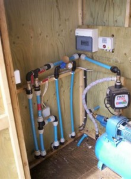
Pumps and Filtration for Private Water Supply, Cornwall
