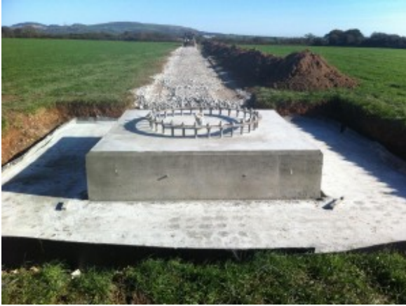
Endurance 50kW Wind Turbine Base
