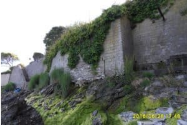
Before :- Sea Wall damaged by storms
