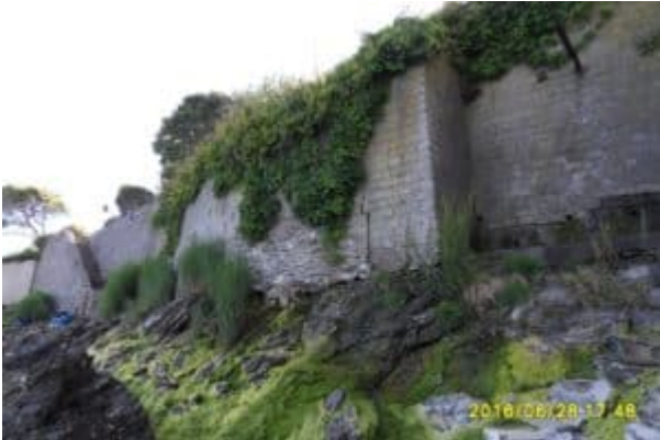
Before :- Sea Wall damaged by storms
